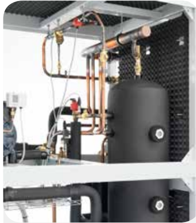
Ricevitore liquido isolato, collettore valvole sicurezza, valvola HPV (in alto) e valvola RPRV. Insulated liquid receiver, safety valve common header, HPV valve (on the top) and RPRV valve.
